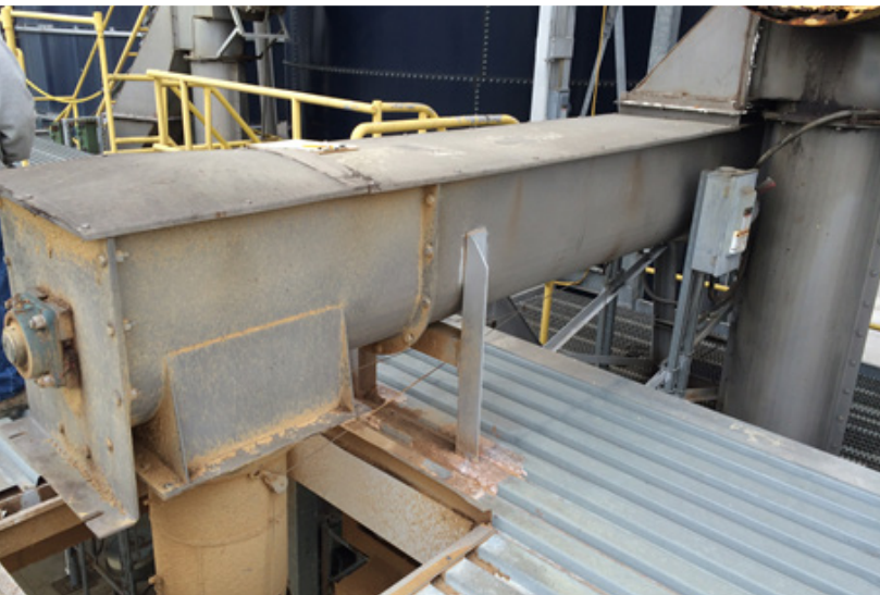
Original Load-Out Screw Conveyor
