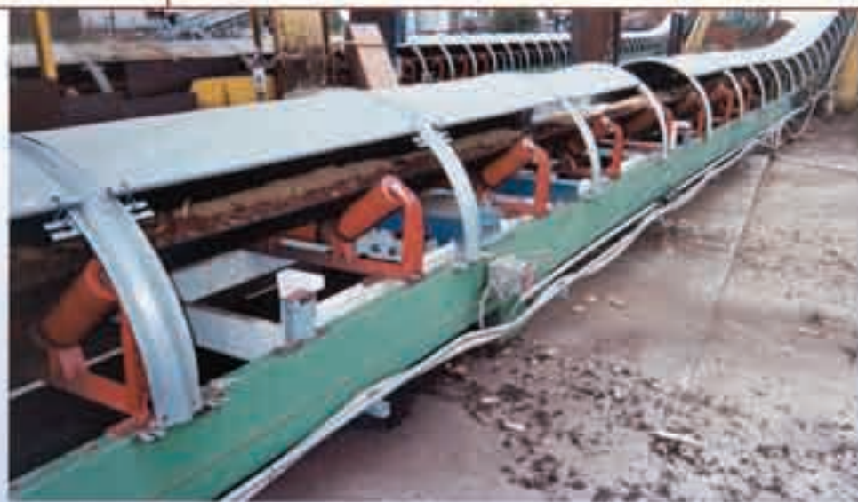
One of two conveyors with THAYER RF (rocking-fixture) belt scales.
